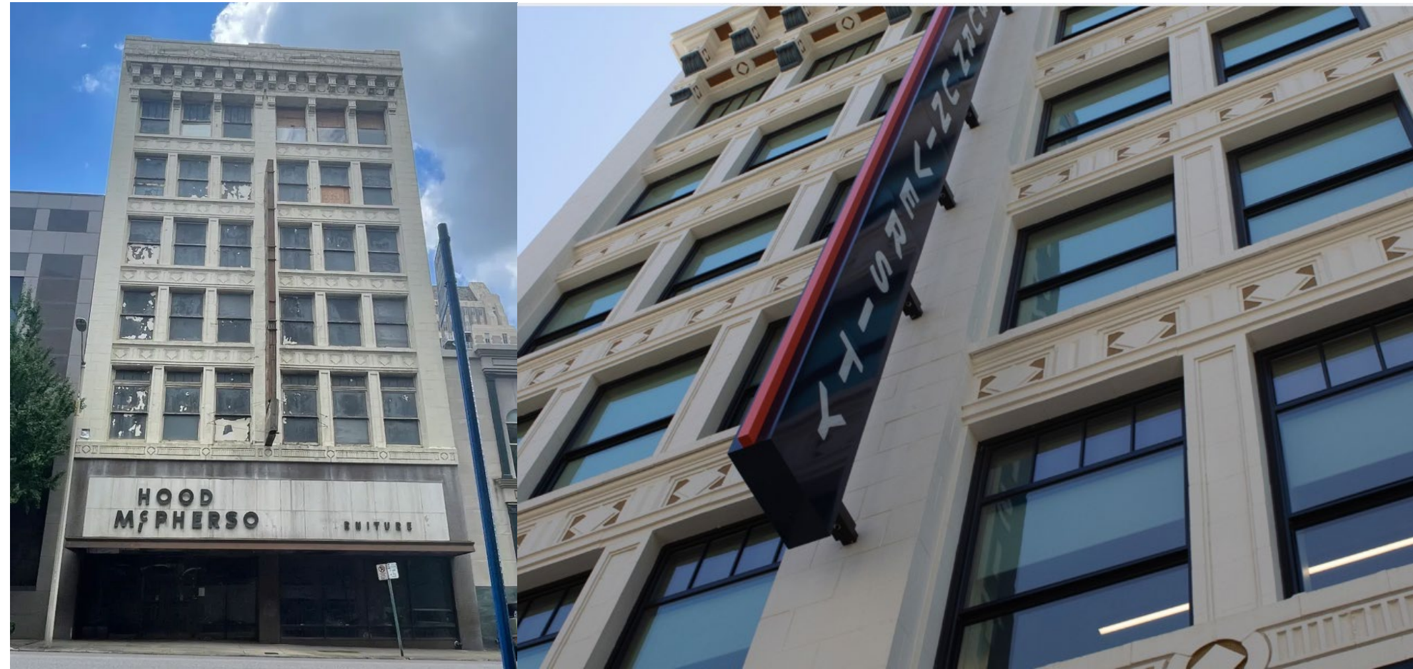
Exterior: Original details were molded, recast, and repainted to keep historic details.
